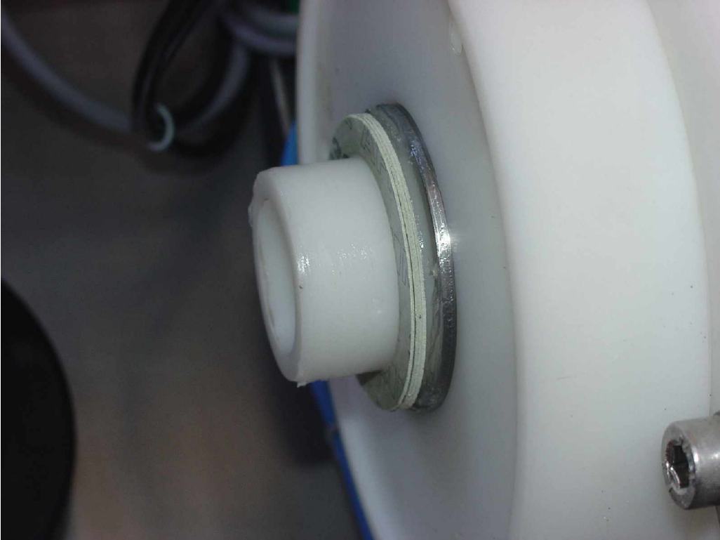
Picture 8 - the rod with the existing intermediate layers. Take off the existing layers.
